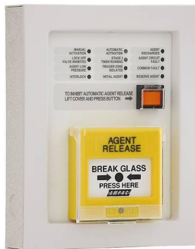
Figure 110: Local Control Station
