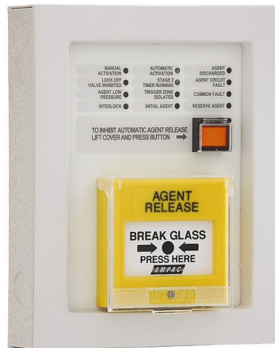
Figure 16: Local Control Station
