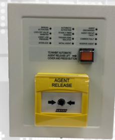
Local Control Station
