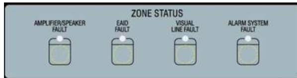
Figure 4: Zone Status Indicators and Switches
